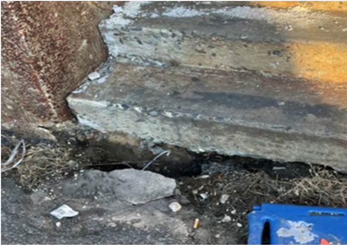
Figure 8. Damaged Base on Dock Step
