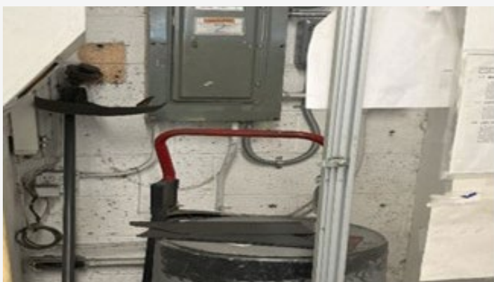
Figure 5. Blocked Electrical Panel
