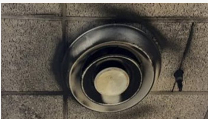
Figure 6. Black Dust On and Around an Air Vent
