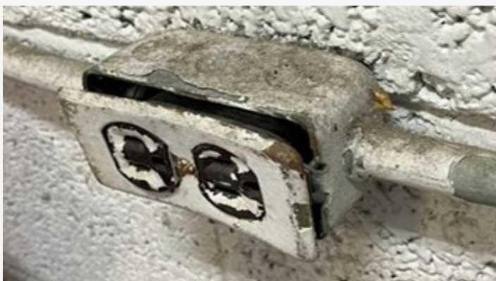
Figure 4. Damaged Electrical Outlet
